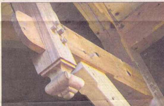
Large pine beams pinned together feature decorative details throughout the timber-frame home being built in St. John's Lake Hills subdivision.
